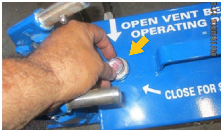
Figure 5.33 - Open Vent on Pump
