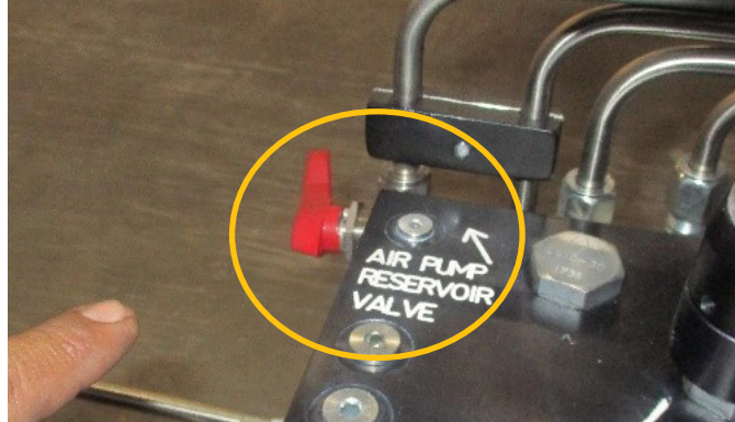
Figure 5.21 - Air Pump Reservoir Valve - Closed
