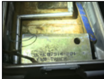
Shipping Spacer Damage
